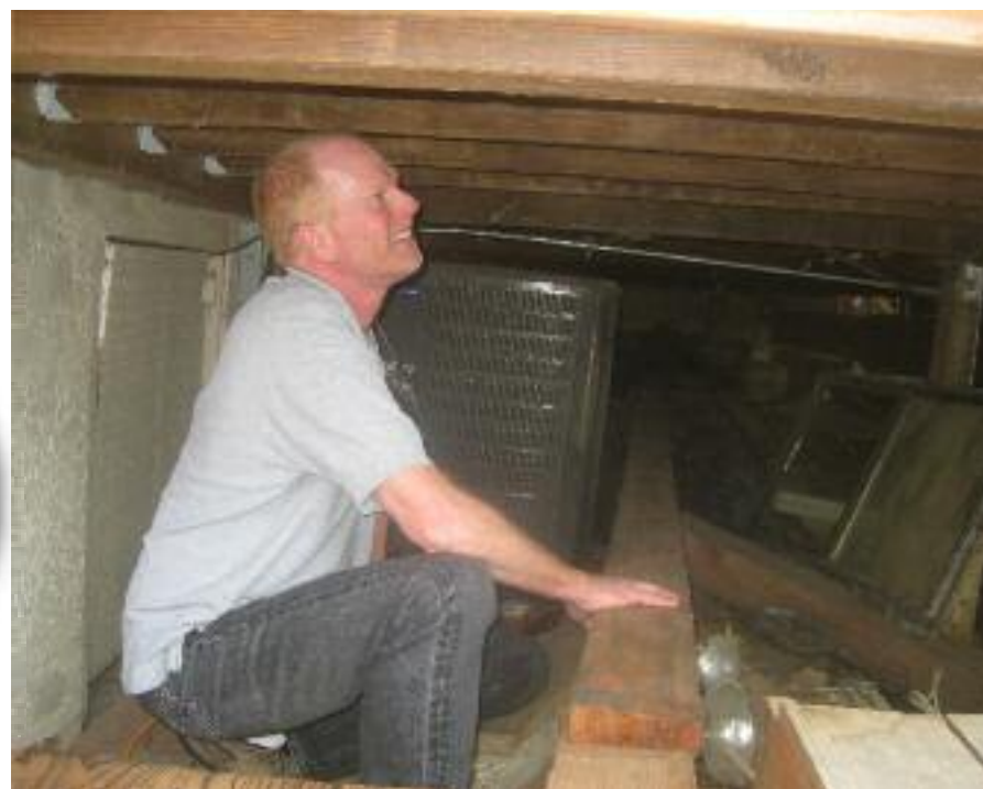
Houghton inspects the under-story of a deck for dry rot.
